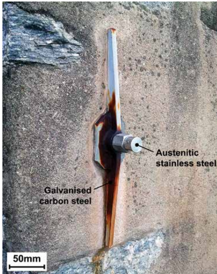
Santa Caterina del Sasso Hermitage , Leggiuno (VA), repair work Tie rod in austenitic stainless steel and frame in galvanized carbon steel Corrosion by galvanic contact in air; temperature range 0°-30°C
